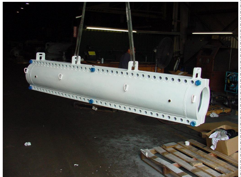
12" ANSI Class 600 – Sub-sea clamp – 10ft long for gas line repair - located at Gulf of Mexico
